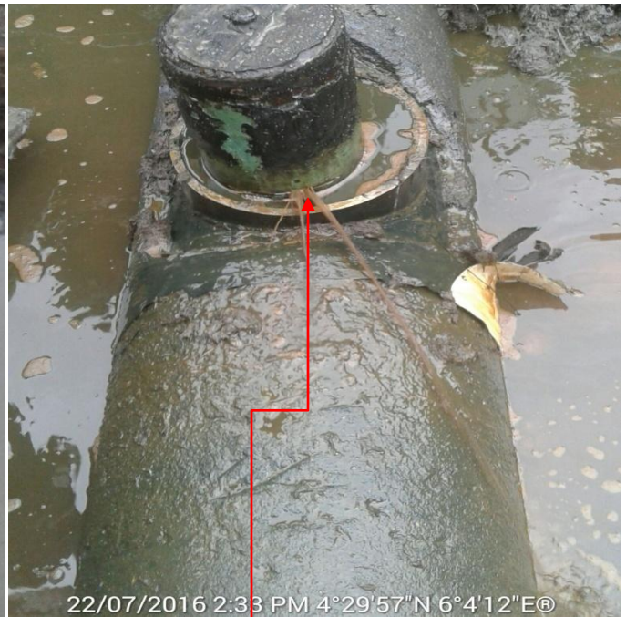
Fig B: The leak point (Hacksaw cut)
